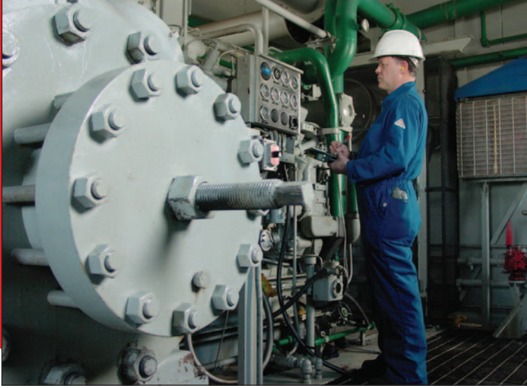
■ A technician checks a 1050 hp FE650D-2 Energy Industries compressor package powered by a Caterpillar G3512TAW engine. This is a 2-throw, 2-stage unit with 16.5 in. (419 mm) and 11.25 in. (286 mm) cylinders in sweet natural gas compression service.
