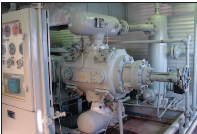
■ This Ajax DPC180 integral is performing better than ever thanks to the Analysis software package. This compressor is in sweet natural gas service, and is a single-throw, single-stage machine with one 10.5 in. (267 mm) cylinder and 171 hp derated for site elevation.
